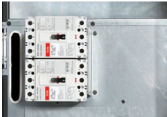
Additional subfeed with aux and shunt trip
